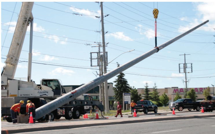
Example of a road closure for hydro pole installation. Poles range in height from 75 to 110 feet.
