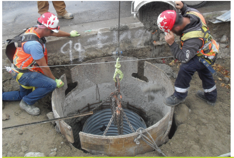
Installing a 4.5-metre deep caisson (hydro pole foundation) on Yonge Street, October 2023.
