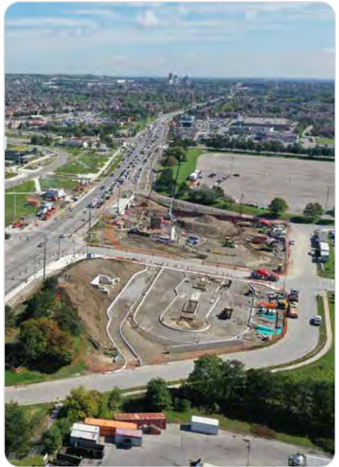
▲ Early phase of construction of Major Mackenzie Drive West bus terminal near Canada's Wonderland in the City of Vaughan.
